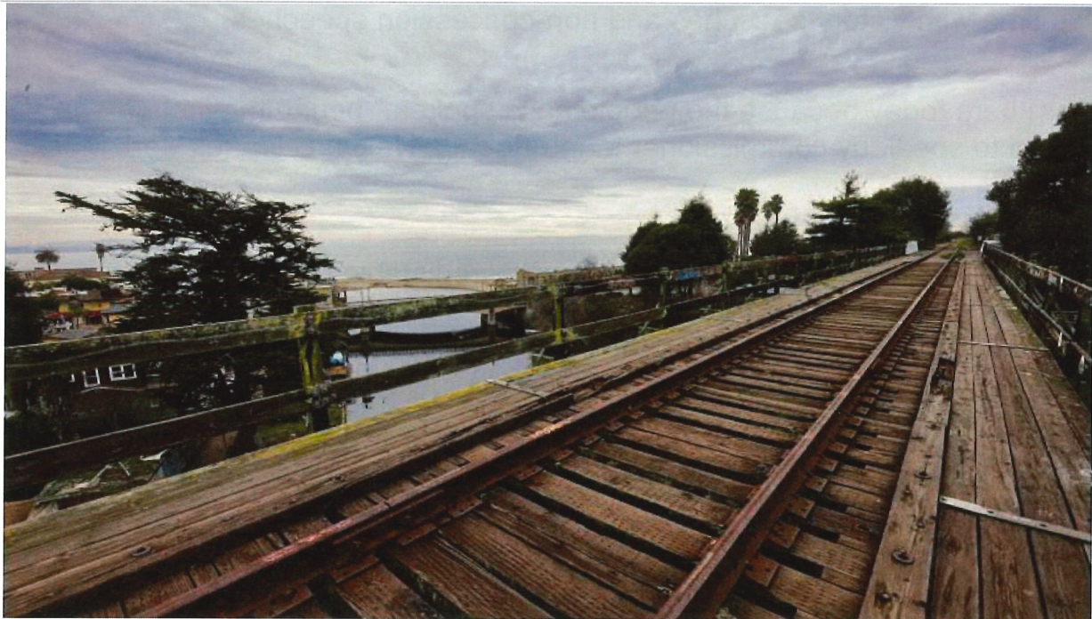
The rail line on the trestle above Capitola Village. (Kevin Painchaud / Lookout Santa Cruz)
